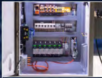
2. System Control Panel
